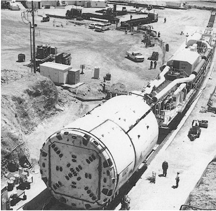
■ ■ Tunnel boring machine. Yucca Mountain Project. (see page 5 of Soils News for details) or http://www.nwer.sandia.gov/ymp/
